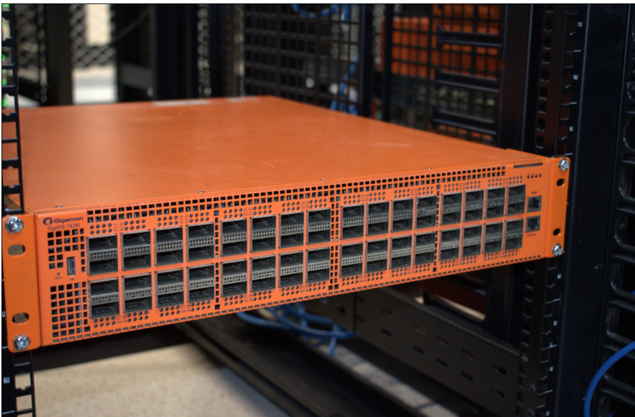
Figure 5 Front View of the Mounted Node to the Four-Post Rack
